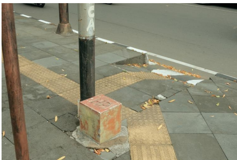
Mis-construction of guiding block paving in the City Walk (Slamet Riyadi St.)
