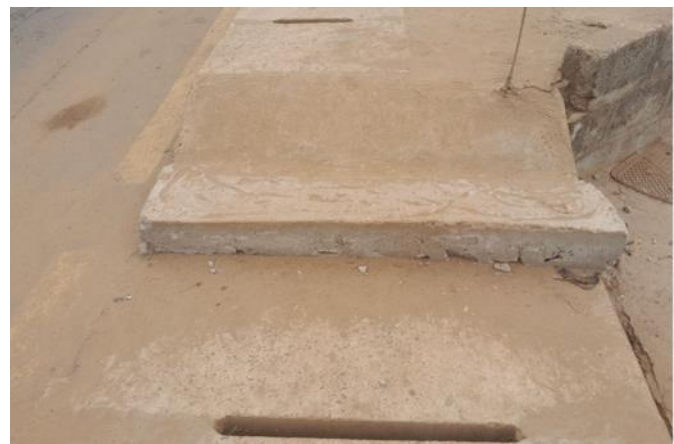
Example of a poorly implemented inclusive design feature
